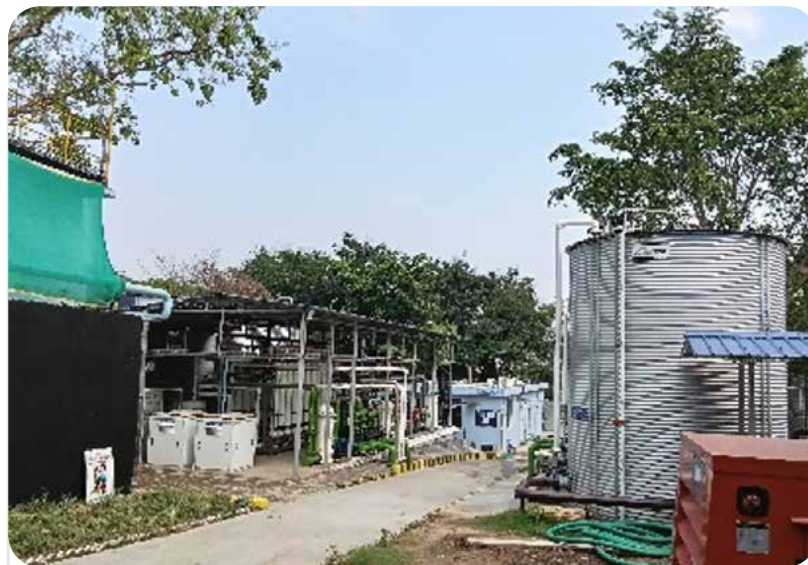
1.6 MLD STP with a 1 MLD UF & RO system set up at Jamshedpur Township supplies treated water for plant.
